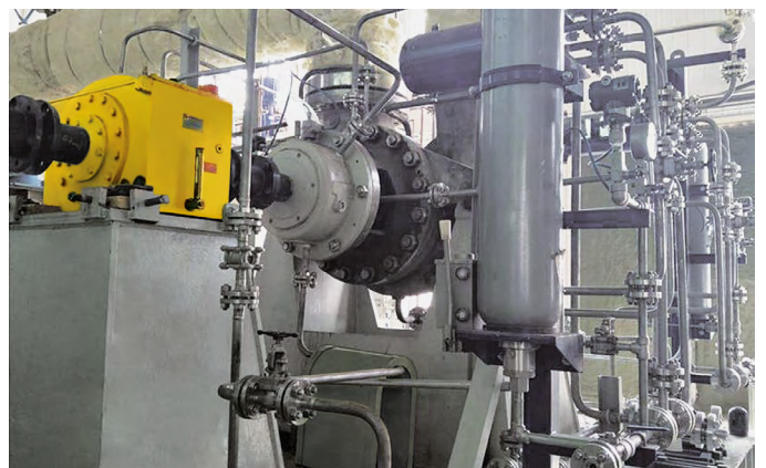
Housing Freewheel FH 4000 in recovery steam turbine
